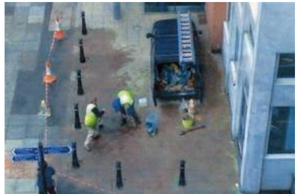
These men have just finished installing the bollards and are clearing up prior to driving away...er...
